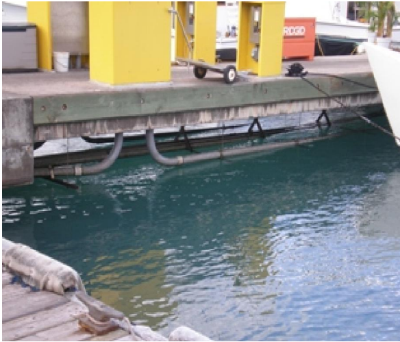
Below water line electrical conduit unsafe
