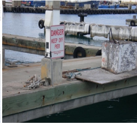
Poor maintenance has led to condemned piers
