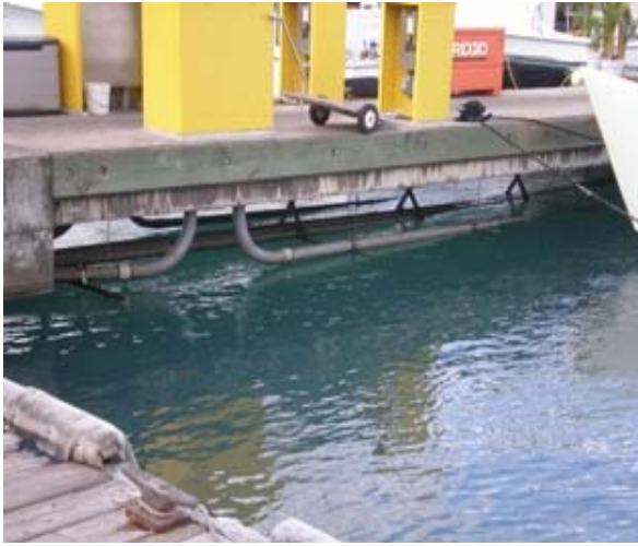
Below water line electrical conduit unsafe
