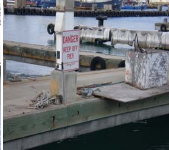
Poor maintenance has led to condemned piers
