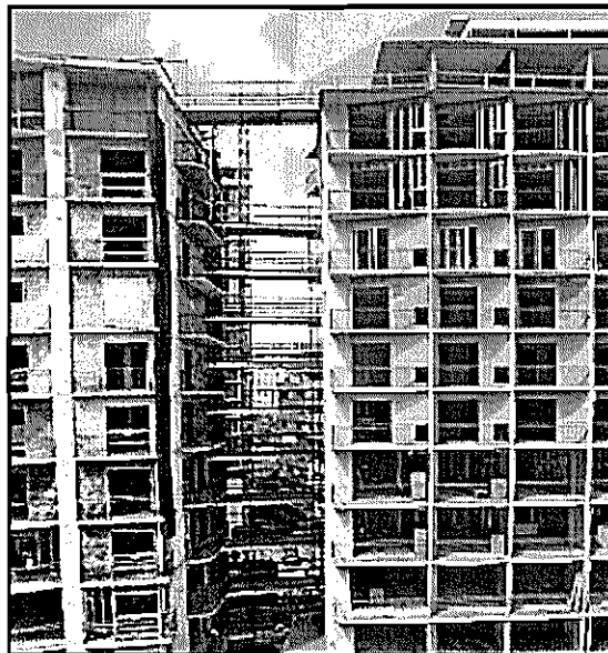
Outrigger's massive Waikiki Beach Walk renovation project is keeping several industry members busy.
