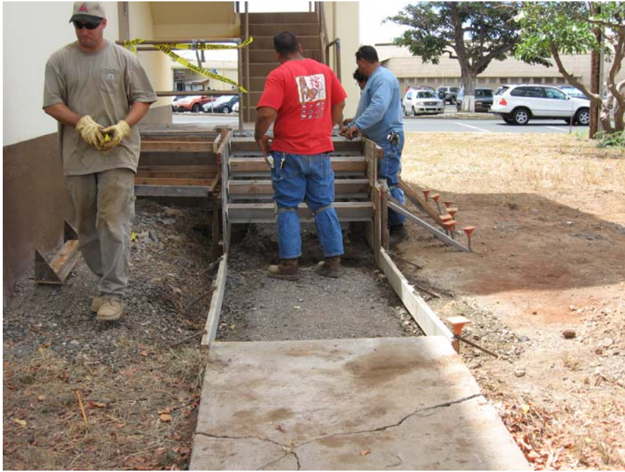
Installation of side forms for new stairway landing and Walkway extension at exterior stair #3.
