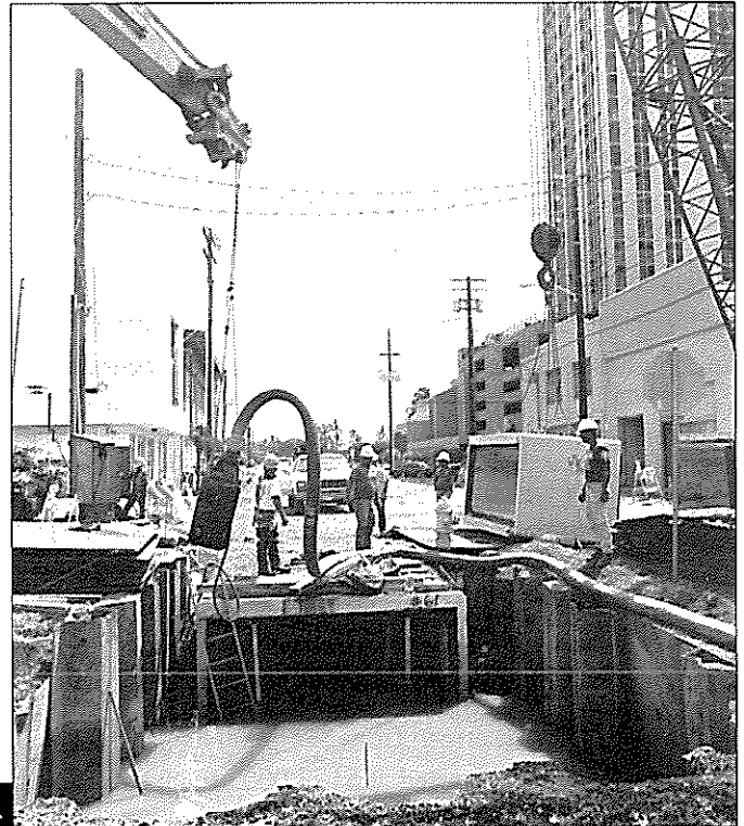
At right, box drains are installed on Kamakee Street near Waimanu Street.
